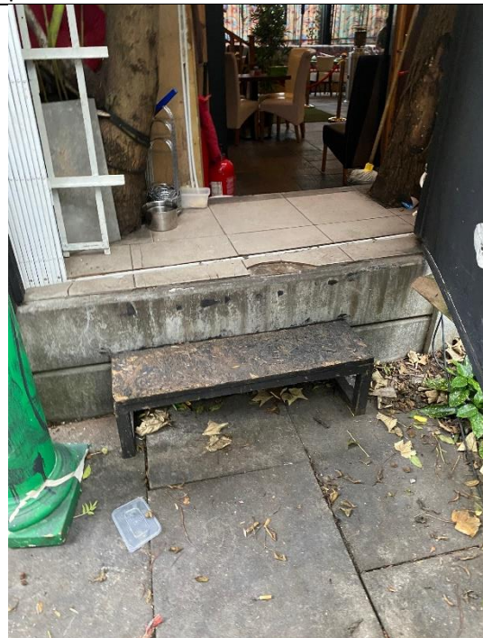
Appendix 7 – Rear fire exit step
